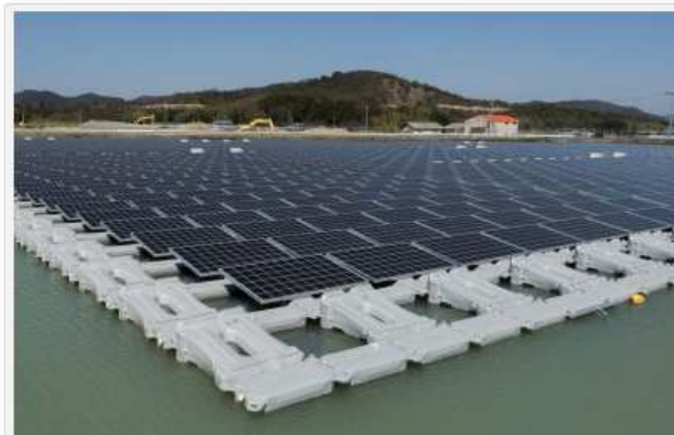
Photo courtesy of Kyocera Kyocera TCL Solar Inaugurates Floating Mega Solar Power Plants in Hyogo Prefecture, Japan
